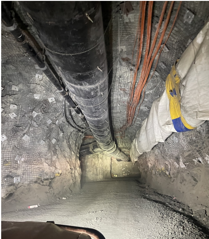
Our ventilation ducting moving air cubes to the face
